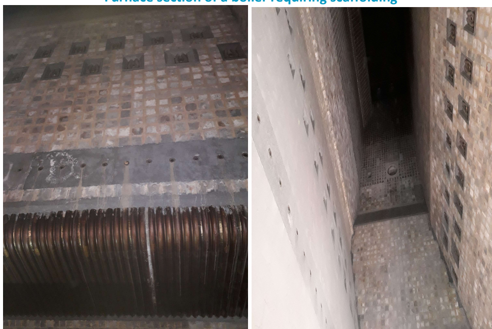
Figure 7-1 Furnace section of a boiler requiring scaffolding
