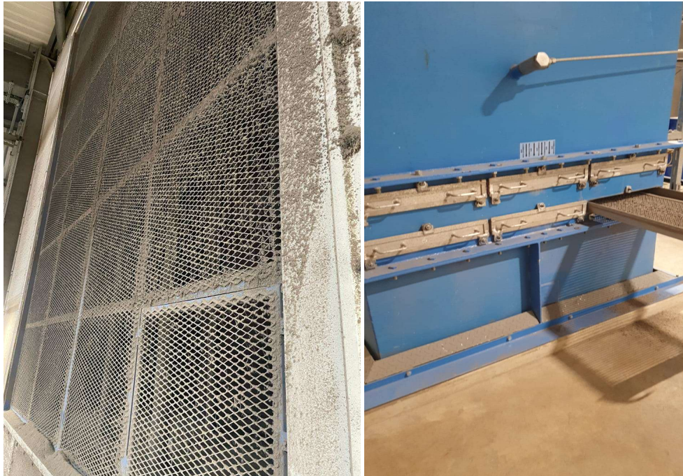
Figure 6-1 Primary air intake in the bunker hall & Figure 6.2 Primary air intake filters
